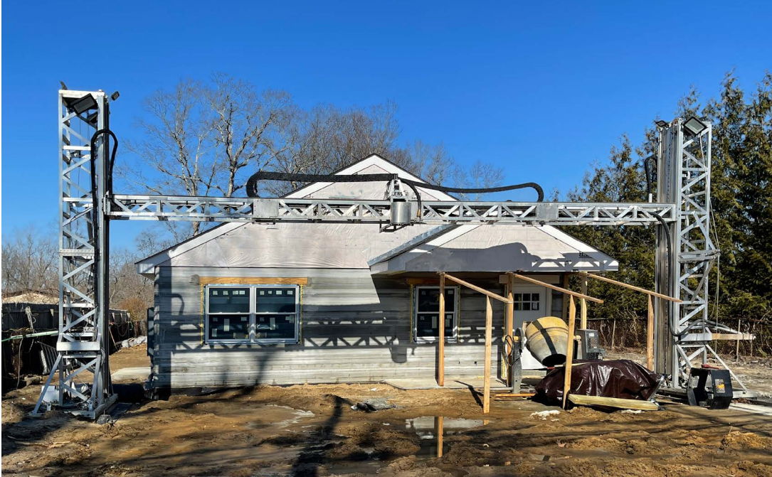
A 3D-printed house under construction in Riverhead, New York (Credit: futurewalk/iStock Unreleased)
